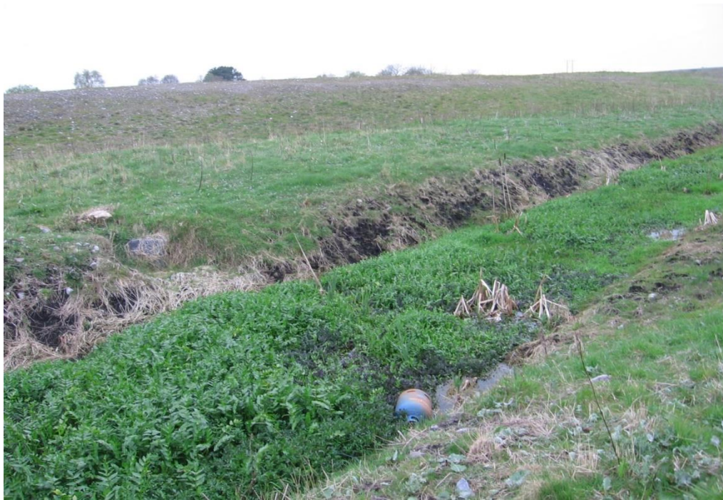
Figure 7.7 - Clogged stream diversion shown at front and peat disposal area in background at Pollboy 3 years after construction
