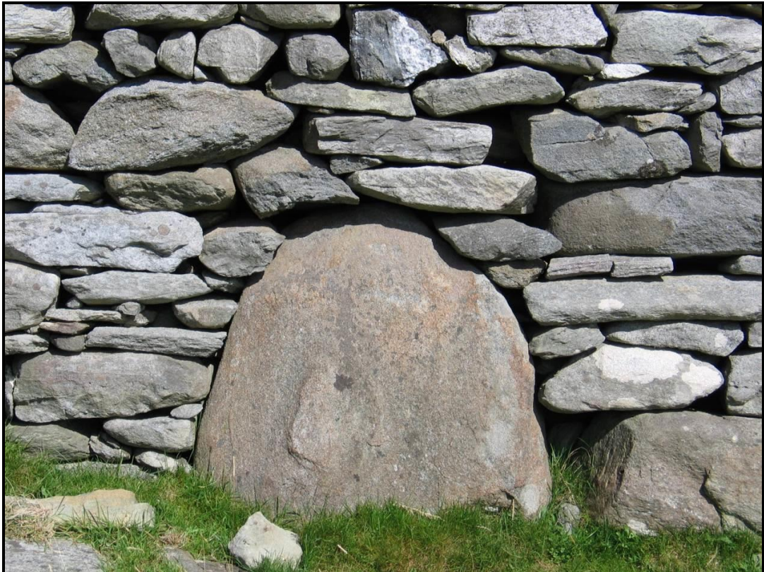
Pl. 95 – House 57 at Slievemore (S57), showing the large curved boulder inset into the wall.
