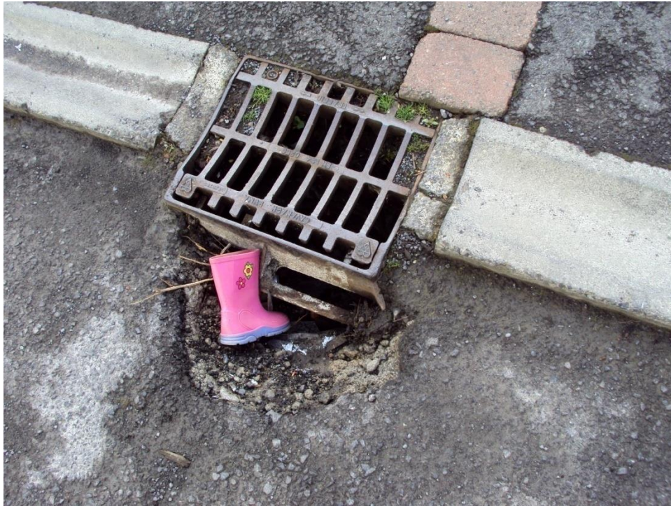
Figure 30 – Dangerous pavements. Photograph FFC Residents Association.
