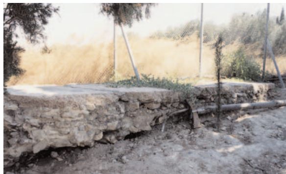
Fig. 1. The remains of a large Roman cistern just north of the Western Court of the Minoan palace.
