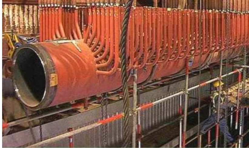
Figure 1.4. Installation of a branched header in ESB power plant (Stephen Scully, ESB Energy International [27]).
