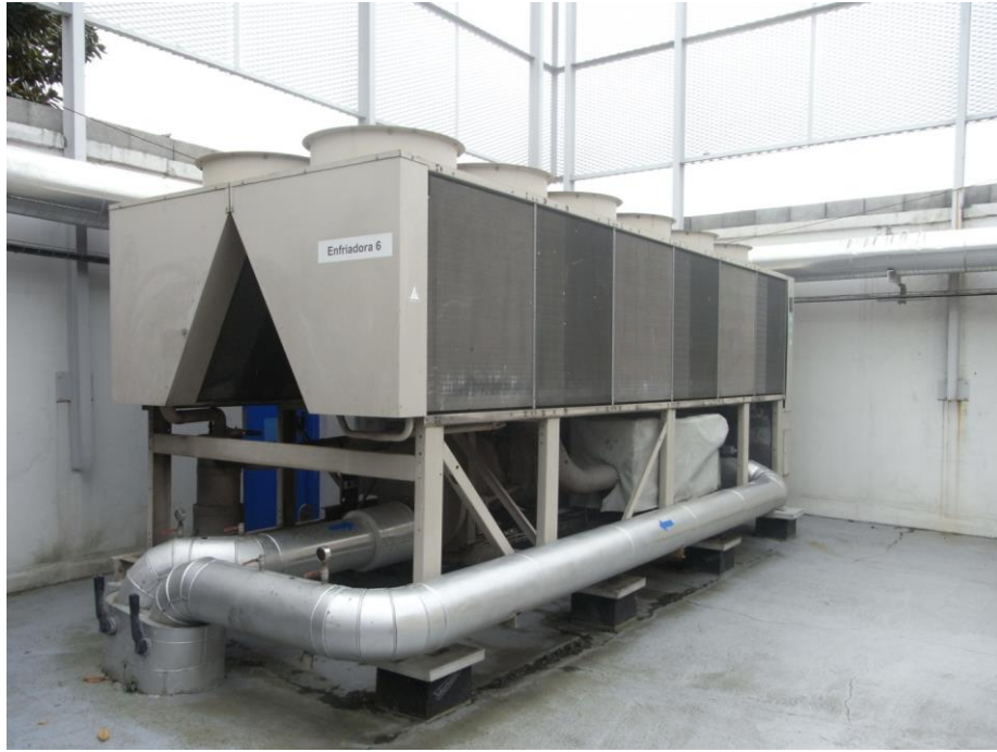
Figure 36. TRANE air-cooled conventional chiller on the roof of the generation plant (Retrieved from INDIGO project [17])
