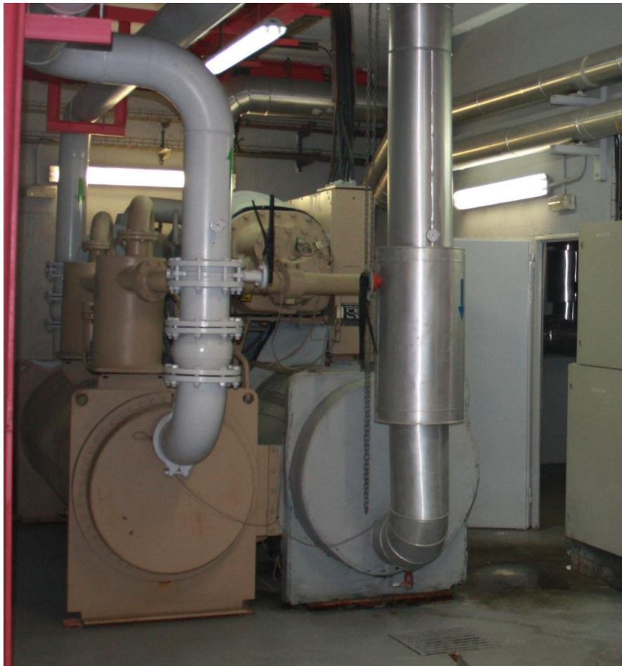
Figure 37. TRANE water-cooled conventional chiller in the generation plant (Retrieved from INDIGO project [17])
