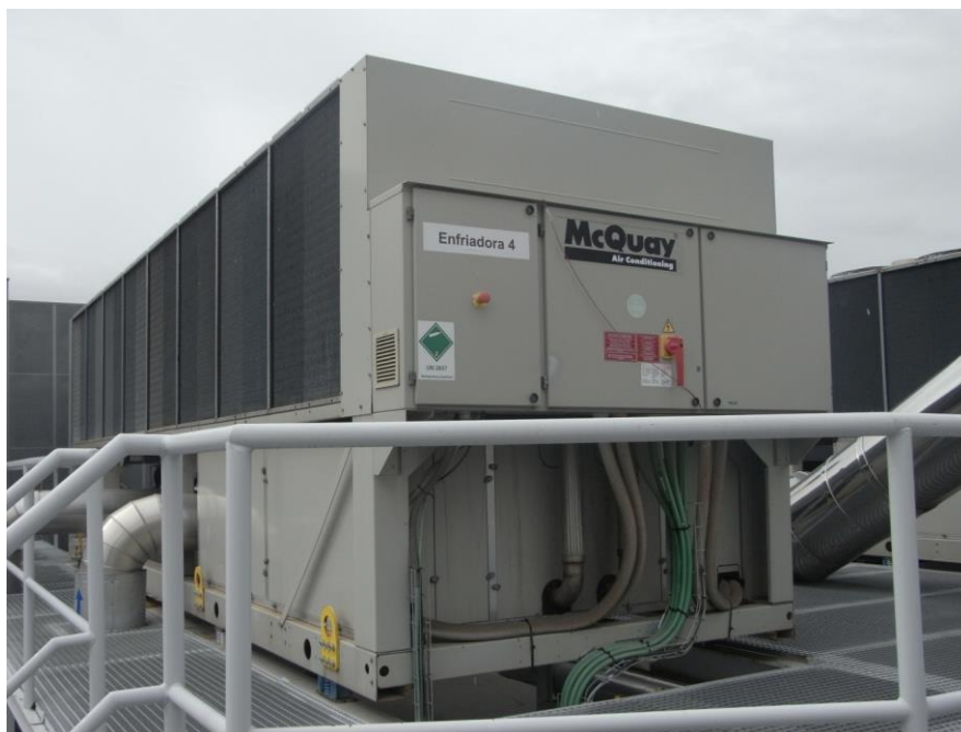
Figure 17: McQuay chiller in Basurto hospital
