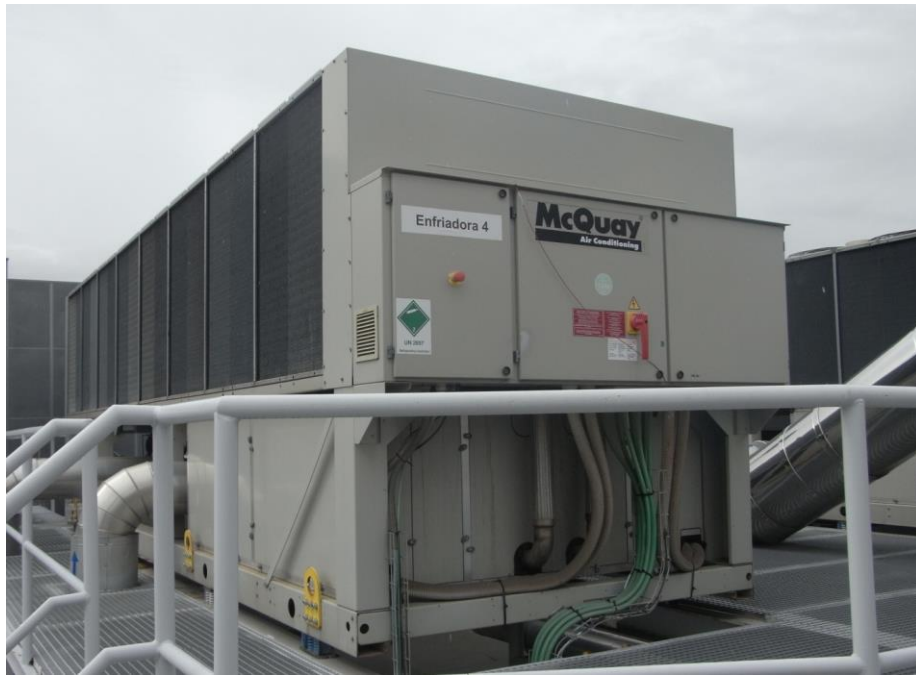
Figure 35. McQuay conventional chiller at its location in the roof of the generation plant (Retrieved from INDIGO project
