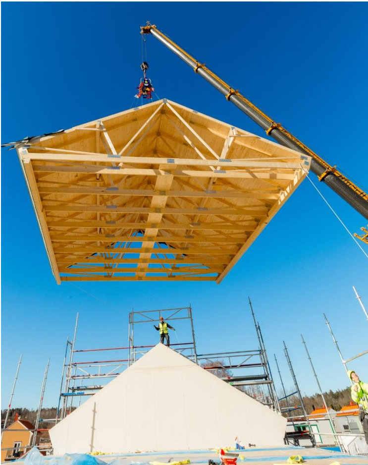
Figure 2-20: Derome roof structure lifted into position on site (image courtesy of Derome).
