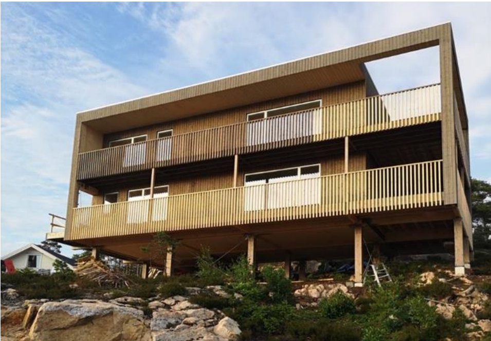
Figure 3-1: The “Villa Forshälla Sund” under construction, in Uddevalla, Sweden (image courtesy of IsoTimber). Designed by Erik Persson and Matilda Lindblom.
