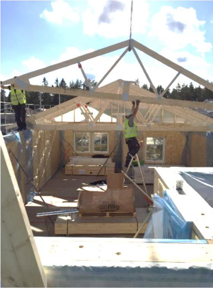
Figure 2-12: Derome roof truss lifted into position on site (image courtesy of Derome)
