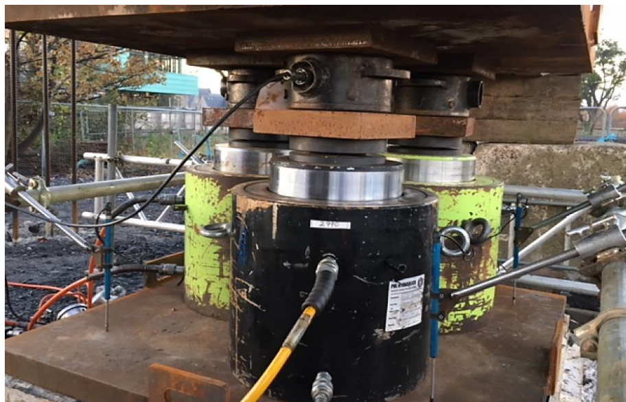
Figure 13. Typical arrangement for (a) static load test with reaction piles, (b) load test instrumentation and (c) multiple hydraulic jacks
