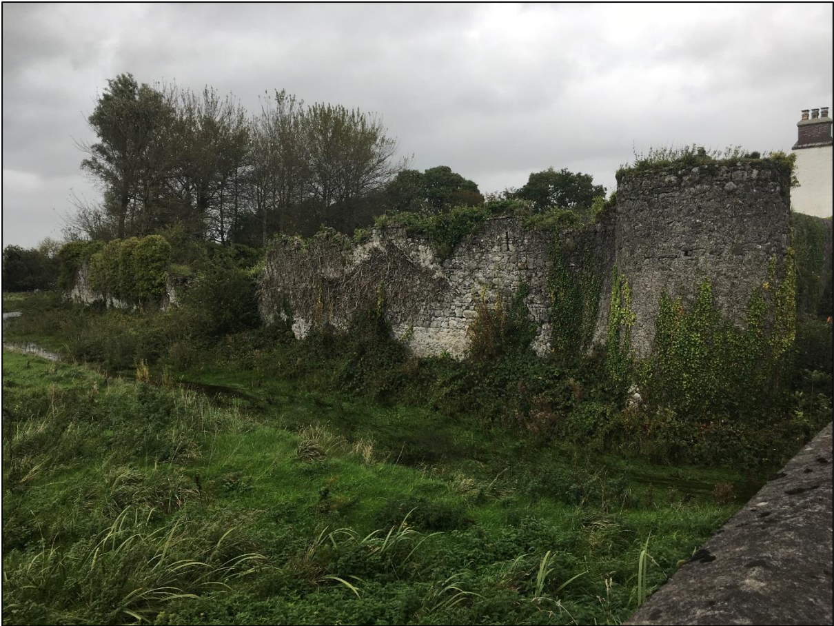
Plate 2 – Bawn wall of the castle (Caislen Suicin) on the eastern bank of the River Suck at Ballinasloe, viewed from the west. Note the repaired wall on the extreme right of the image, and the partially filled remains of a wet ditch on its western side. (Author's photograph)
