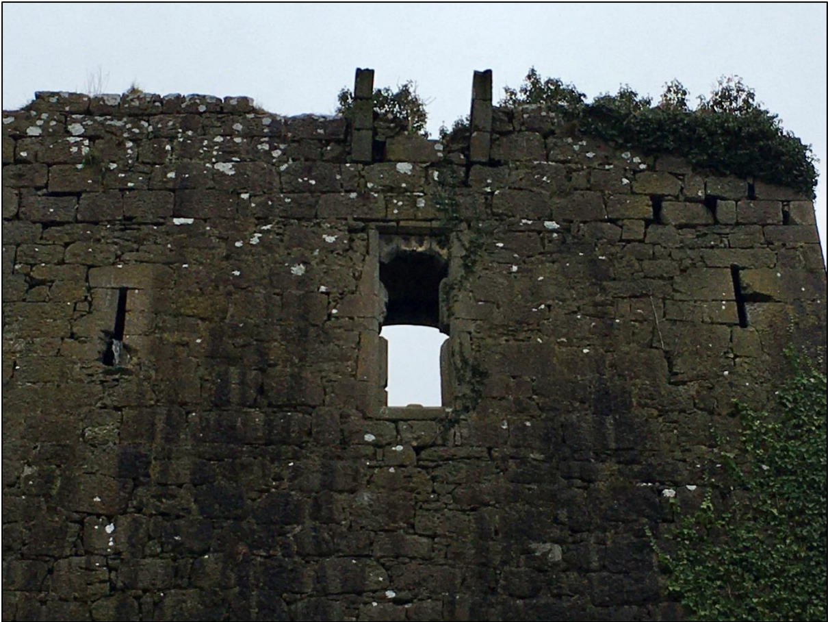
Plate 7.12 – The two light ogee-headed window on the north-eastern wall of the tower house lighting the second floor, flanked by two narrow loops. Note the remains of a possible machicolation over this window, presumably accessed from the battlements on the roof of the castle (Author's photograph).
