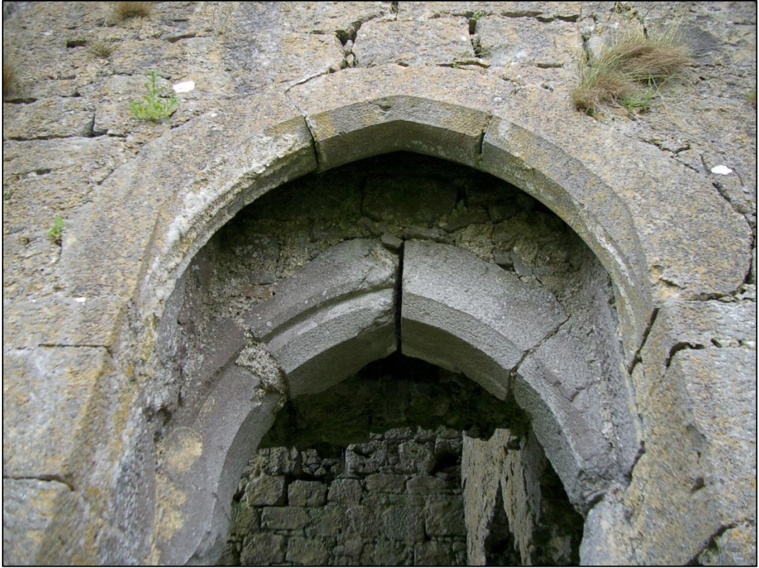
Plate 7.11 - Original pointed doorway of Garbally Castle, Co. Galway (Image courtesy of Mike Salter).
