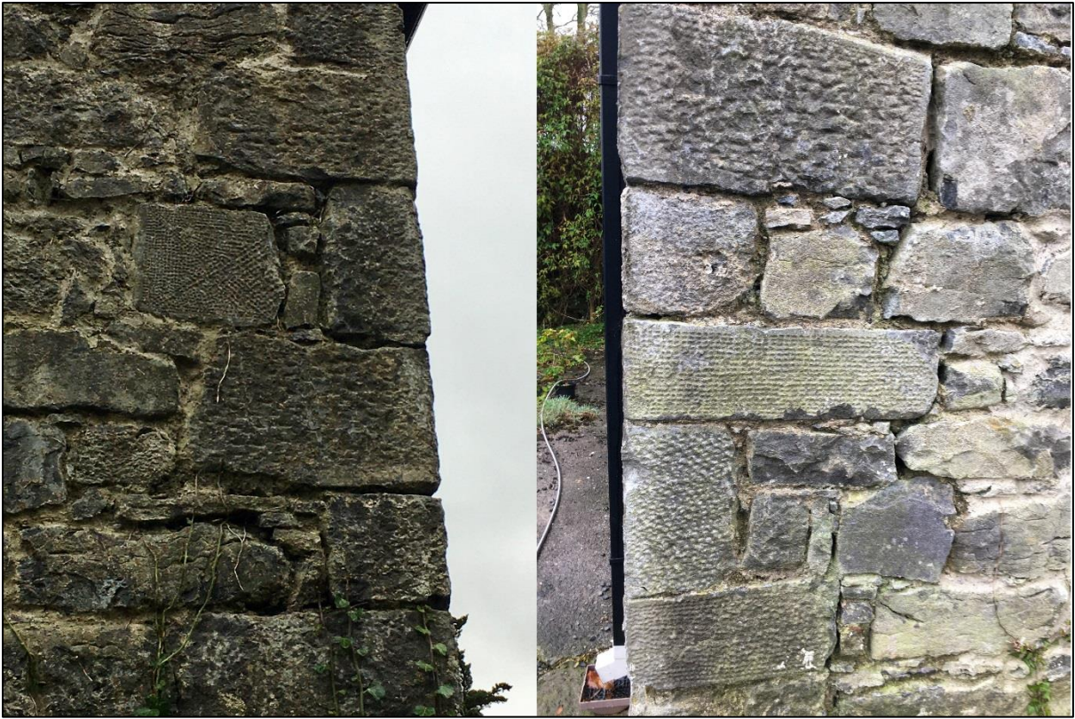
Plate 7.4 – Some examples of the range of punch-dressed stones, including quoin stones, which have been incorporated into the building fabric of the eighteenth-century estate house of Sandfield House. In a number of instances, the punch-dressing is finely tooled in its pattern, which may be an indication of the skill of the masons employed to construct Lisdaulan Castle, and a sign of the wealth of the occupants (Author’s photographs).
