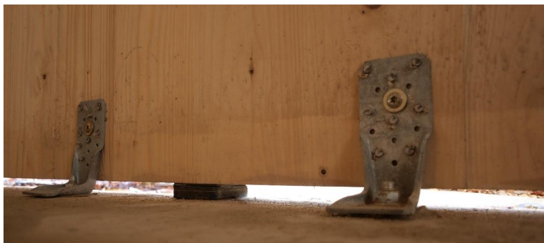
Figure 5.7 Hold-down brackets in-situ, Bishop's Stortford, UK. A 10 mm gap is maintained between concrete ground floor and vertical timber wall panel.
