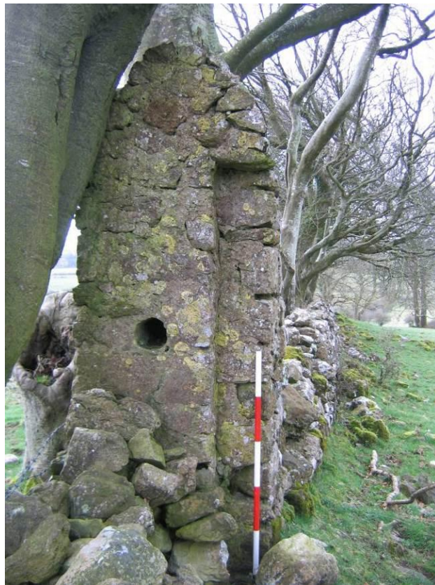
Pl. A5.27: Southern wall end viewed from the north, showing the central aperture and the western recess in the wall end
