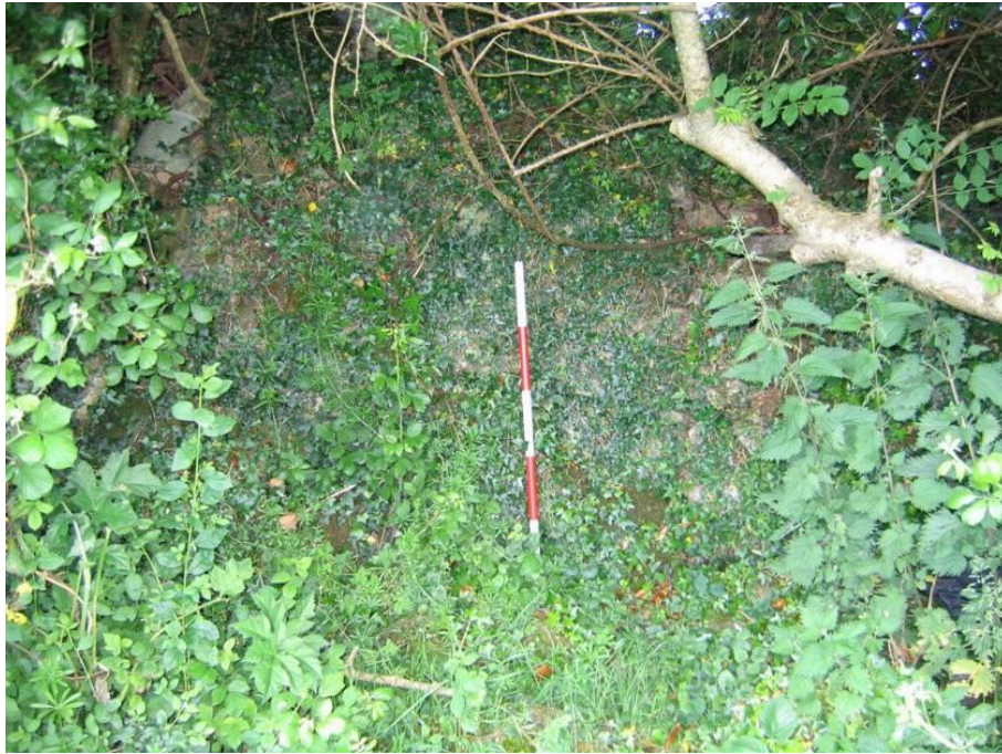
Pl. A5.6: 3m of bank with 1.8m+ of wall forming a revetment, E7
