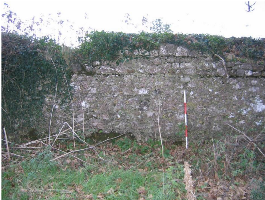
Pl. A7.12: Wall running alongside the road. Three phases are visible, D24
