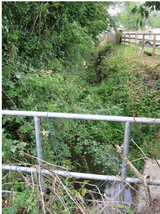
Pl. A6.6: Looking northwest from the Moyglare Road. The ditch is c. 2m-2.5m deep and c. 3m wide, M10
