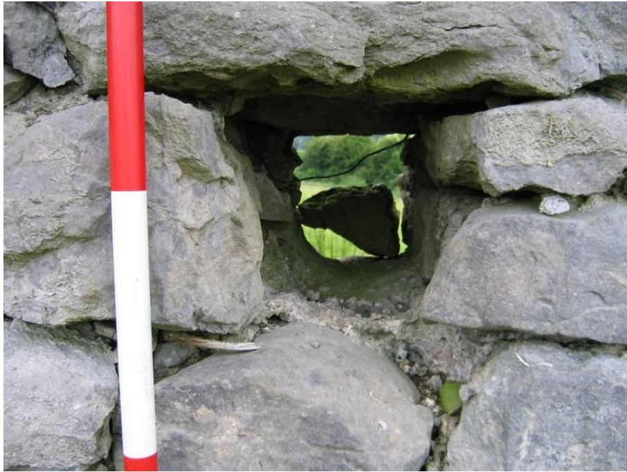
Pl. A5.22: Taken from outside the townland boundary. Close-up of the rectangular hole in the wall, E30
