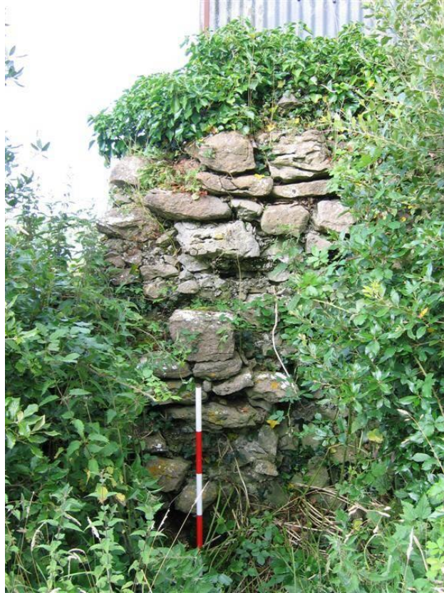
Pl. A5.2: High section of wall at cattle shed (from outside townland) showing 1.8m of original wall topped by modern repair, E2
