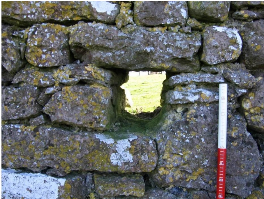
Pl. A5.23: Taken from inside the townland boundary. Close-up of the rectangular hole in the wall, E30
