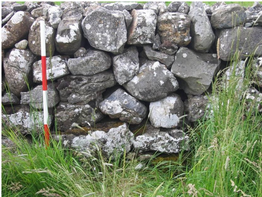
Pl. 5.2: A rebuilt stretch of wall, with one probably original course surviving at the base immediately to the west of E43
