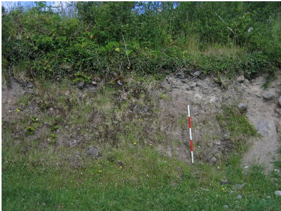
Pl. A5.7: 2.5m+ of vertically sided bank topped by a 1m modern wall, E8
