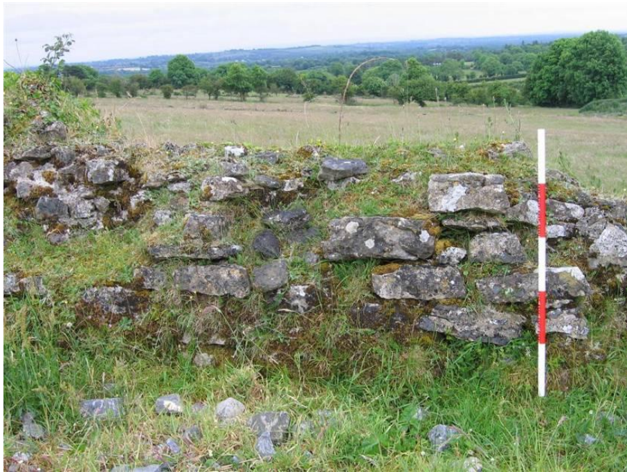
Pl. A5.19: Original wall immediately to the east of the track, E26
